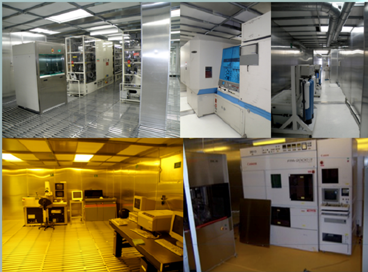
RTP and conventional Furnaces Critical dimension measuring system including ellipsometer and resistivity mapping system installed at INAOE.
